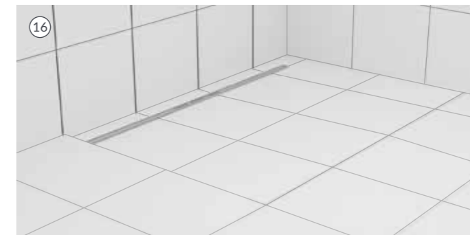
16. Leave for the minimum time recommended by the manufacturer (1.5 h only for the WIPER Tanking Kit) and proceed with the tiling work.
